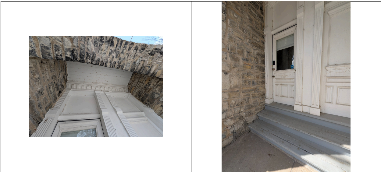
Left: paint cracking and buildup on door panel. Right: non-historic hardware and accumulated paint on door and pilaster.
