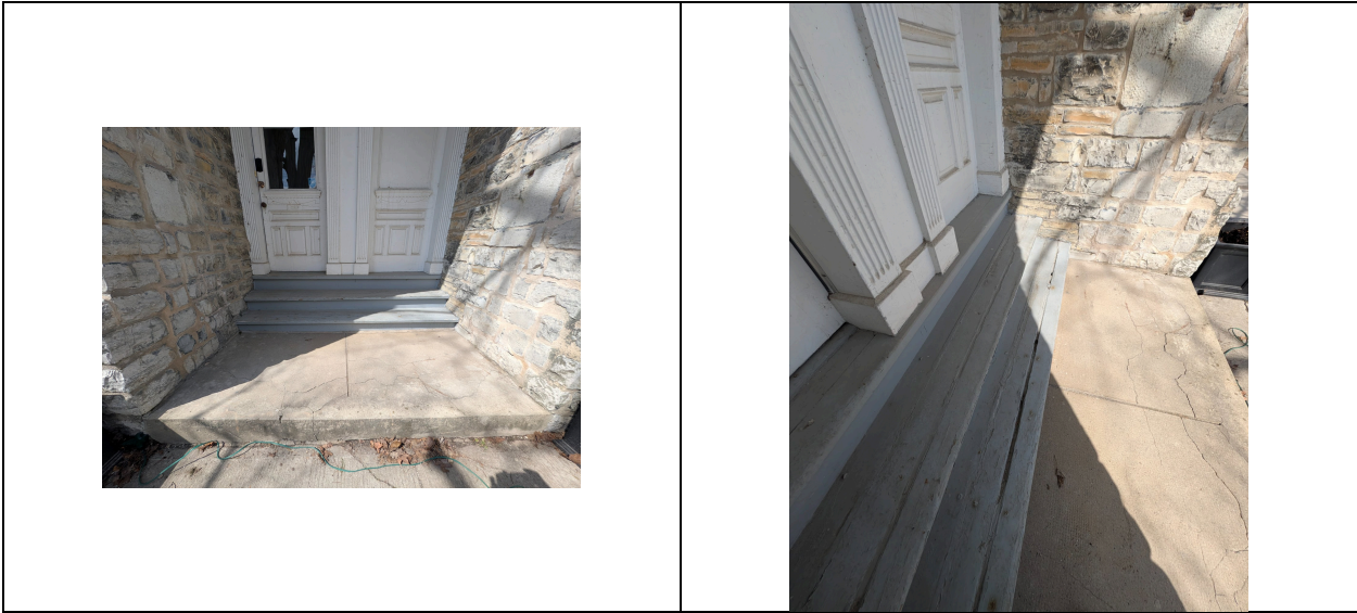
Left: cracked concrete landing pad. Right: deteriorated wooden step treads.
