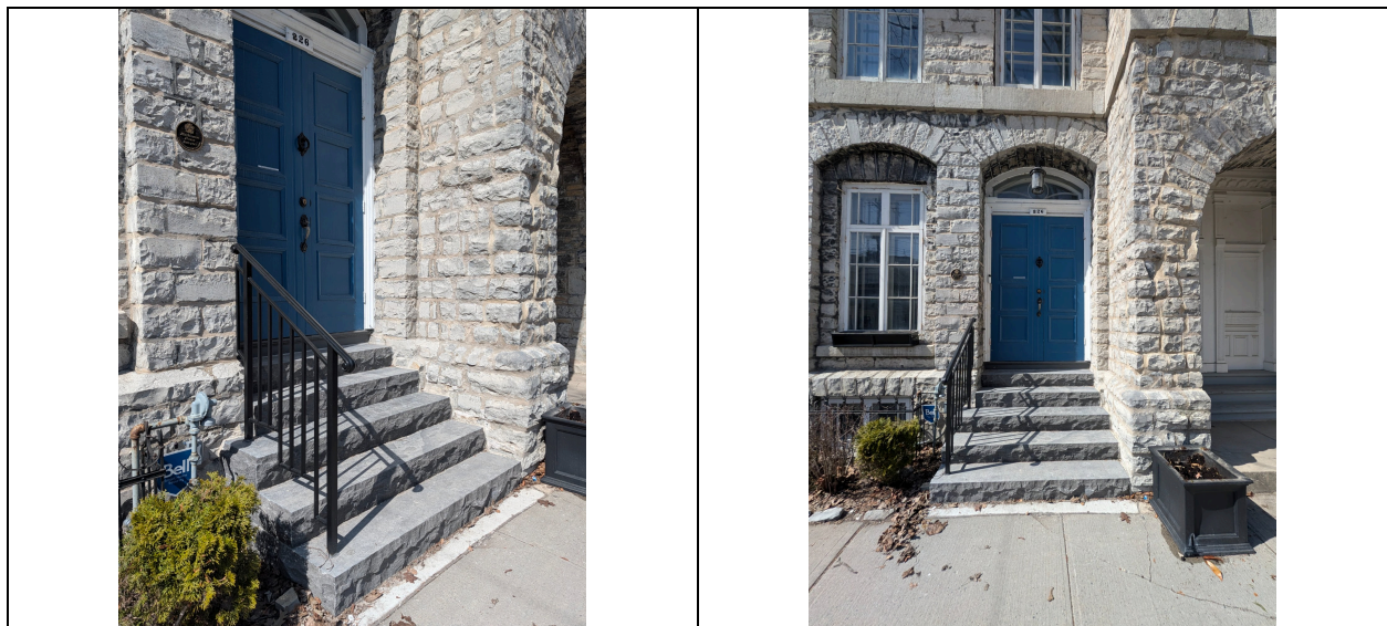
Phase 2 completed: new limestone steps and wrought-iron railing at the main entrance (2025).
