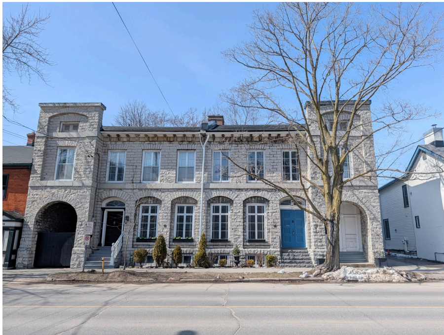
Full façade of Muckleston House, showing the infilled carriageway bay (right) contrasted with the intact original carriageway on the adjoining property (left).
